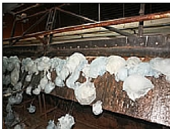
Figure 28. Jellyfish clogging the cooling system of a power plant.
