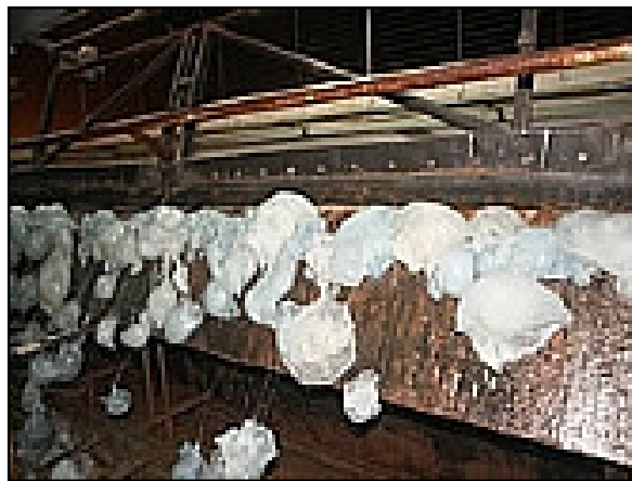
Figure 28. Jellyfish clogging the cooling system of a power plant.
