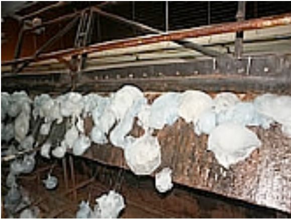
Fig. 28. Jellyfish clogging the cooling system of a power plant
